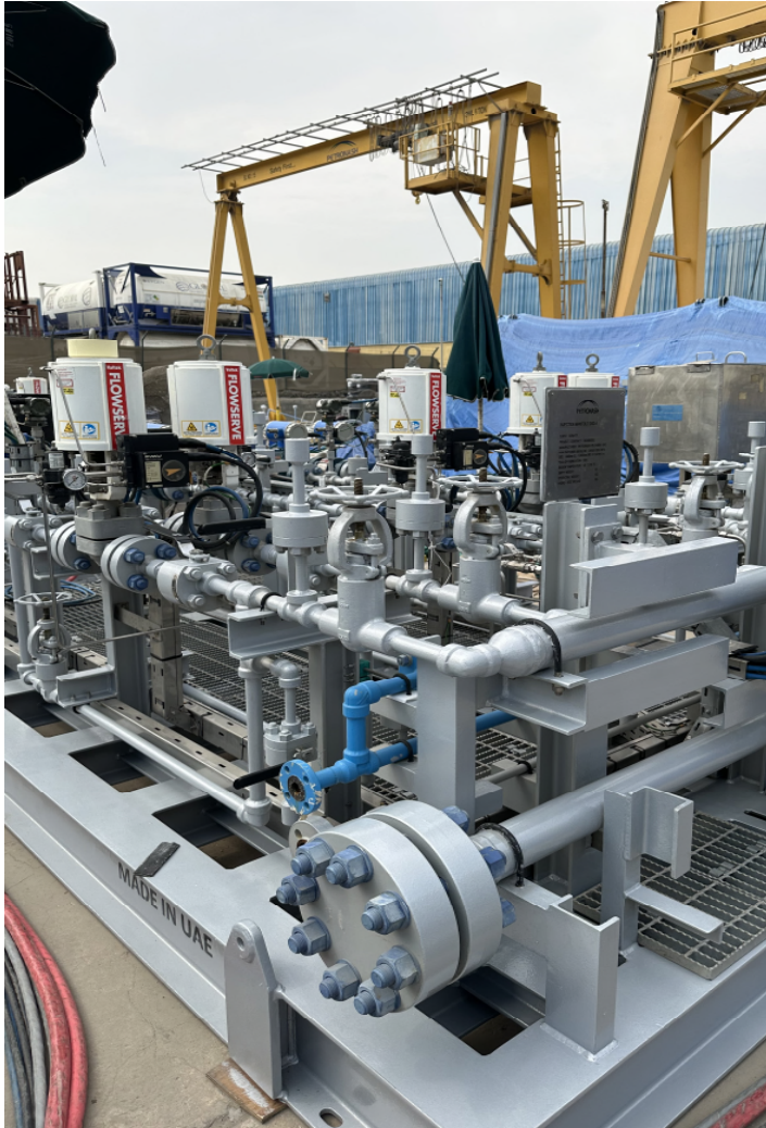
Finger Manifold SKID
