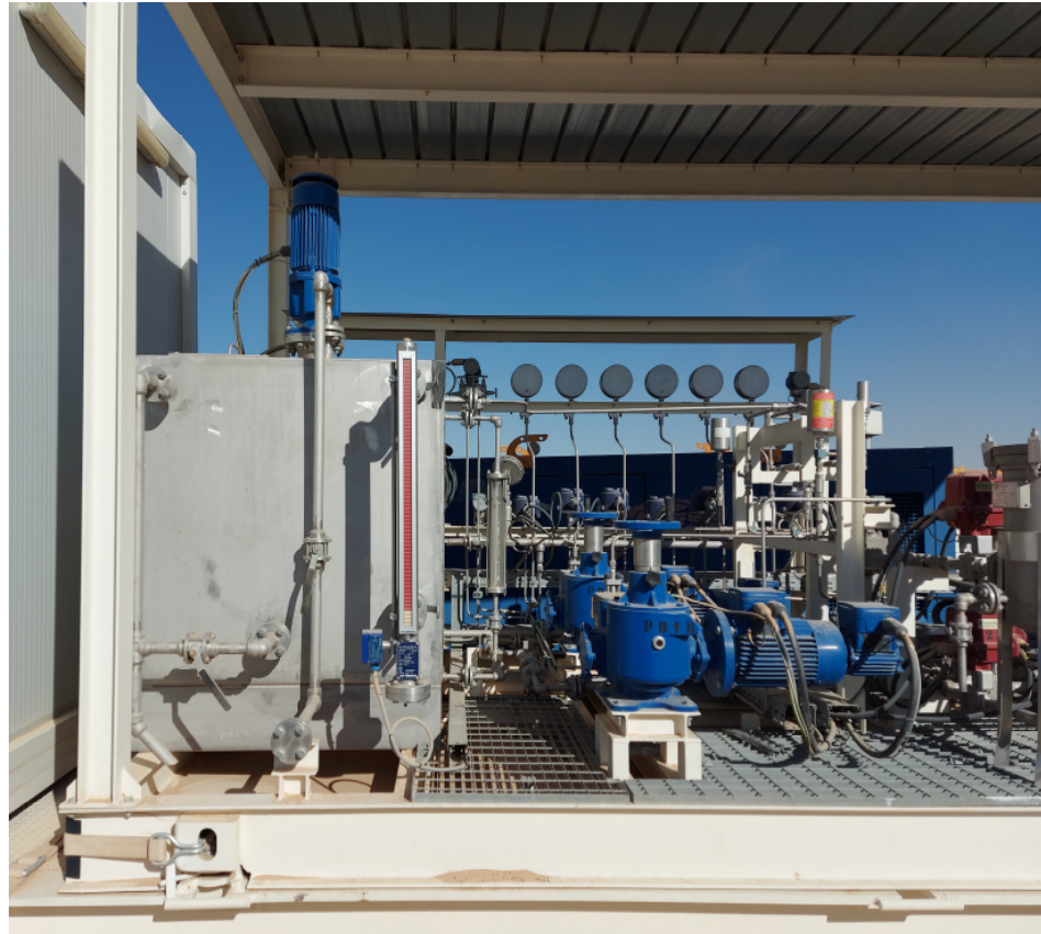
Chemical tank with agitator
